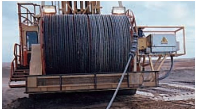
Cavotec reel on a surface drilling machine, USA
