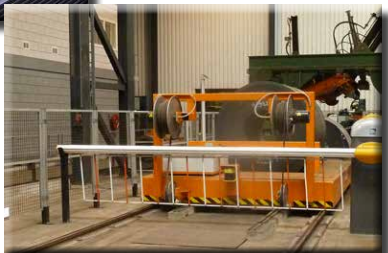
AV40 cable reels for feeding and controlling of a transfer cart and machines
